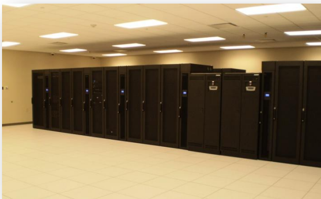
The new Licking Memorial Hospital Data center
