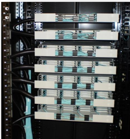
Fiber Enclosure Installed at the LMH data center
