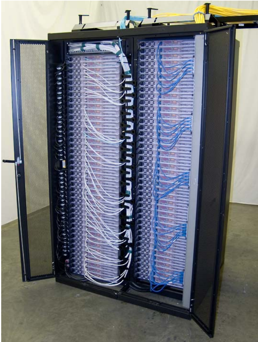
Figure 1: Comparing Vertical Patch Panels to Standard Patch Panels in Server Applications
